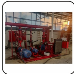
Fire Fighting Pumps
